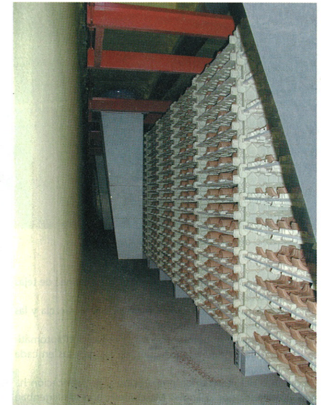
Interior secadero "baladoblic" lateral
